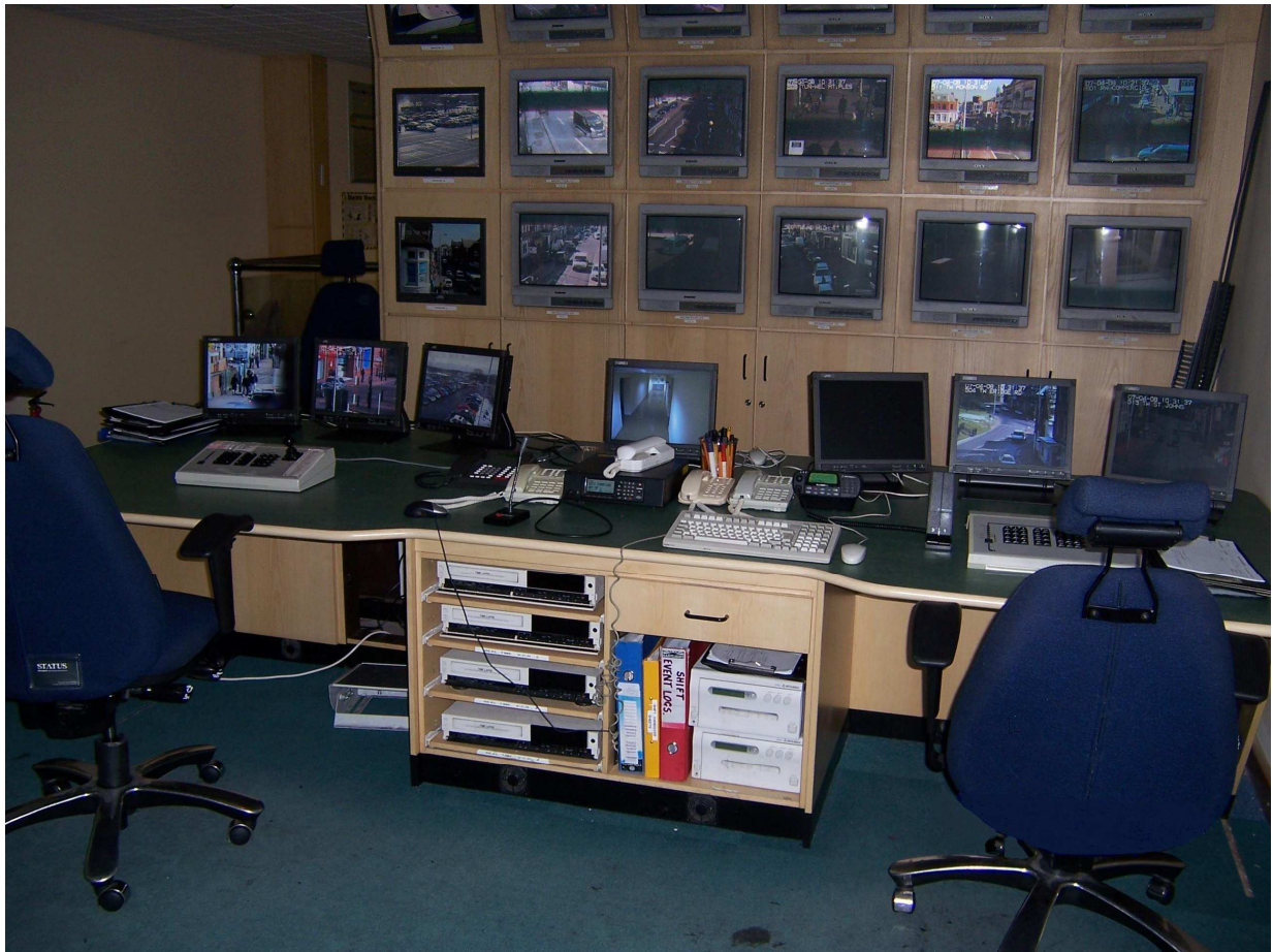
CCTV Control Room
